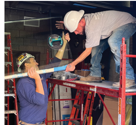
Dariusz Trochim and Gilbert Morales, glaziers with Talisen Construction, hoist a glass plate into its frame at Abrons Arts Center.
